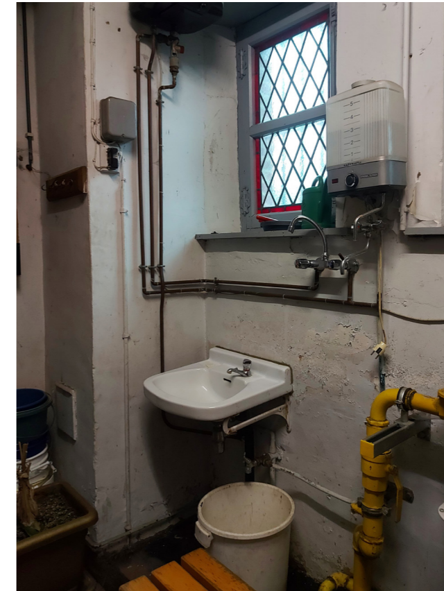
wastafel in depot
